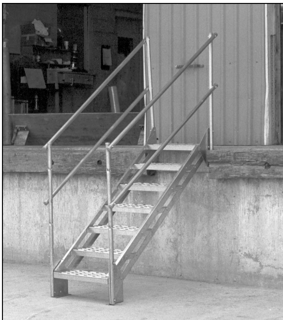
Typical application of stairs, complete with hand rails.
